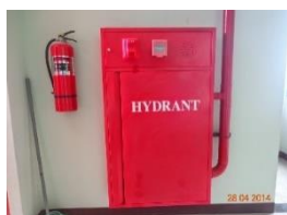
Gambar 95. Hydrant Box & APAR
