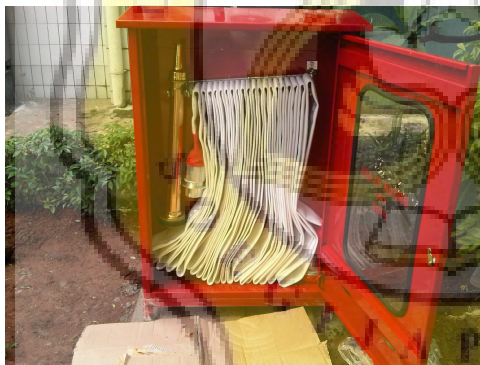
Gambar 73: Kotak Hydrant (Sumber : www.americanwatercollege.org )
