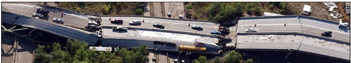
Figure 1. The Mississippi Bridge Collapse, August 2007 (taken August 5 from www.telegraph.co.uk .)
