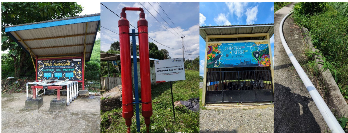
Picture 10. Facilities for methane gas energy in Manggar Final Waste Disposal Site (Source: own picture)
