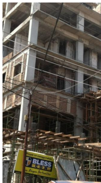
Picture 6. The demolition of Tjan Bian Thiong for the development of Amaris Malioboro Hotel (source: gudeg.net).
