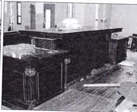
Figure 2 12 Catholic Church damage in Temanggung
