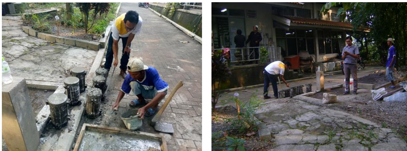
Figure 10: Mixing a concrete stir for a concrete cylinder test (left) and making a concrete test specimen (right)
