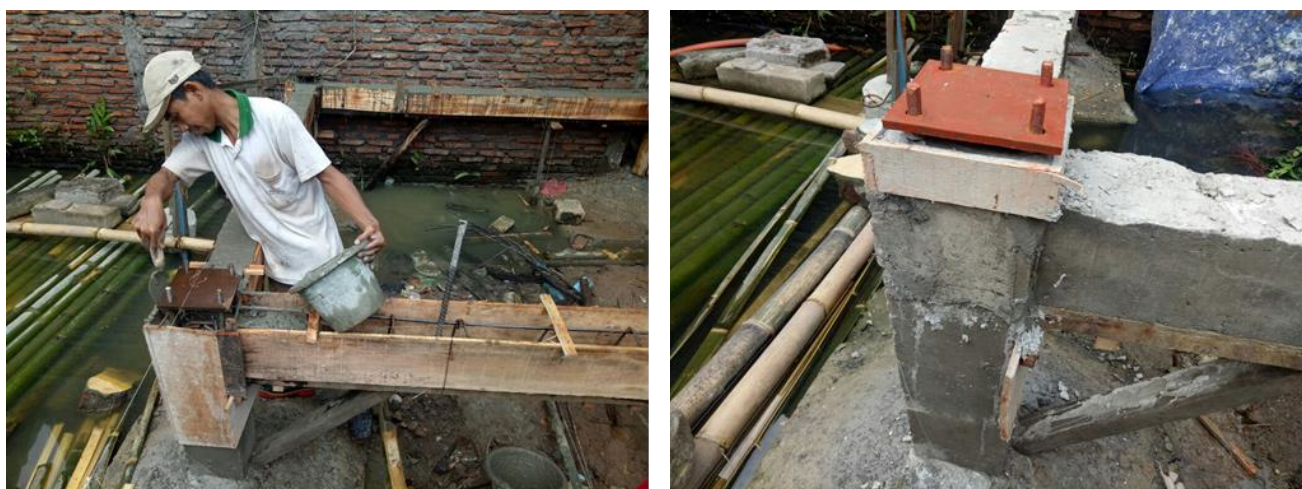
Figure 9: Casting of sloof beam and raft foundation column (left) and finished casting of sloof beam and raft foundation column (right)
