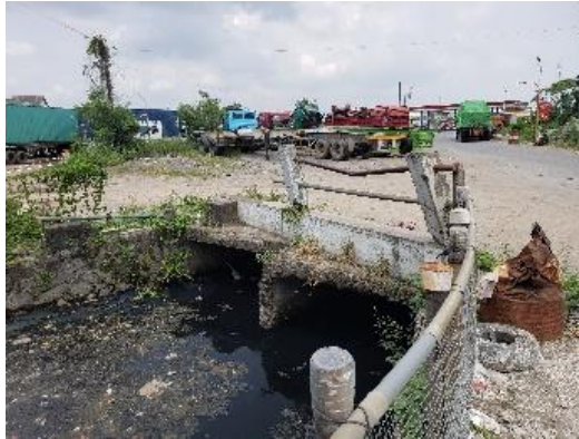
Gambar. 8 Kondisi Sarana Prasarana & fasilitas- Drainase
