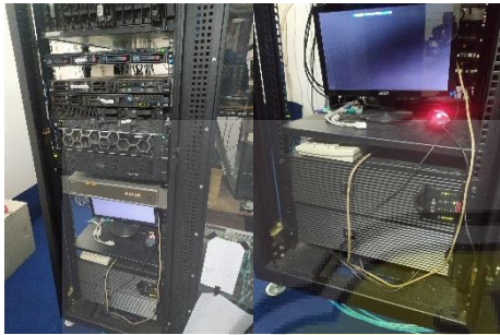
Gambar 5 Rak Server Data Center Unika
