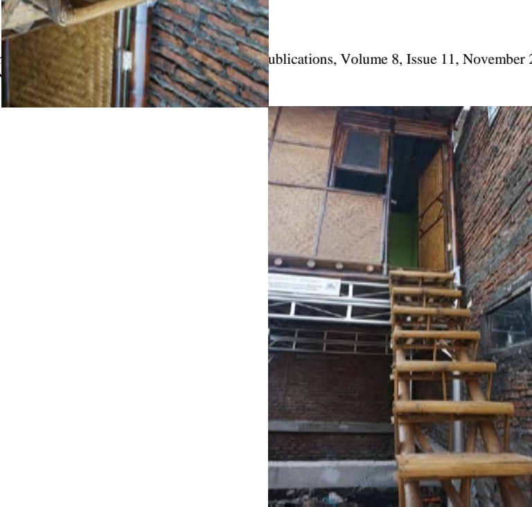
Figure 6 : The stairs to the stage house made of bamboo
