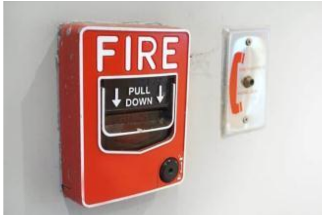
Gambar 7.6 Fire Alarm (sumber : Google Image)
