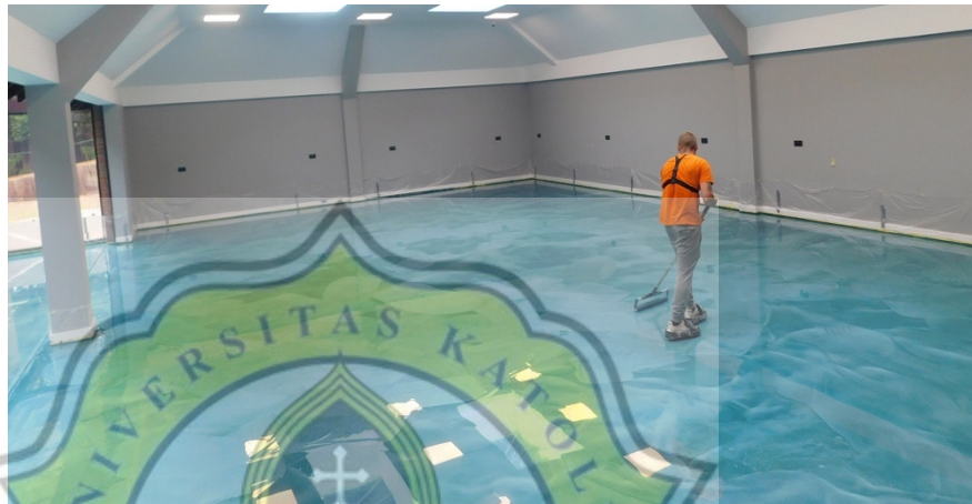
Figure 41. Epoxy flooring (Source: www.jenflow.com )
