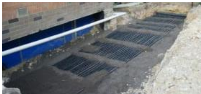
Gambar 65 In Ground Water Tank
