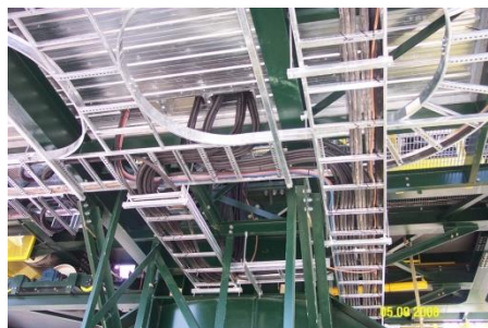
Gambar 32. Wiring Installation Sumber : google.com
