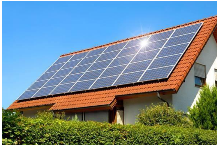
GAMBAR 66 Panel surya (sumber : google image)
