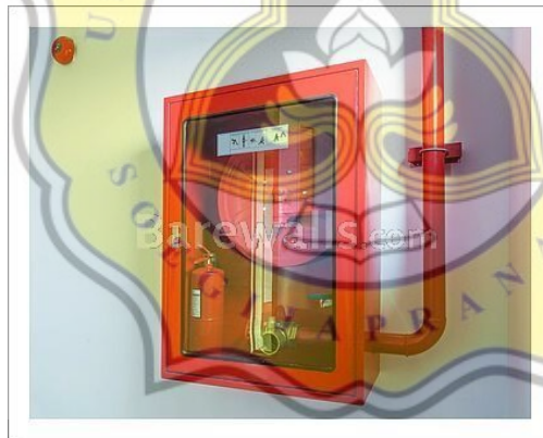
Gambar 7. 29 Indoor box hydrant Sumber : barewalls.com
