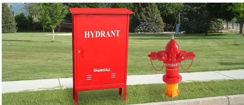
Gambar 7. 30 Outdoor hydrant box dan hydrant pillar Sumber : bromindo.com
