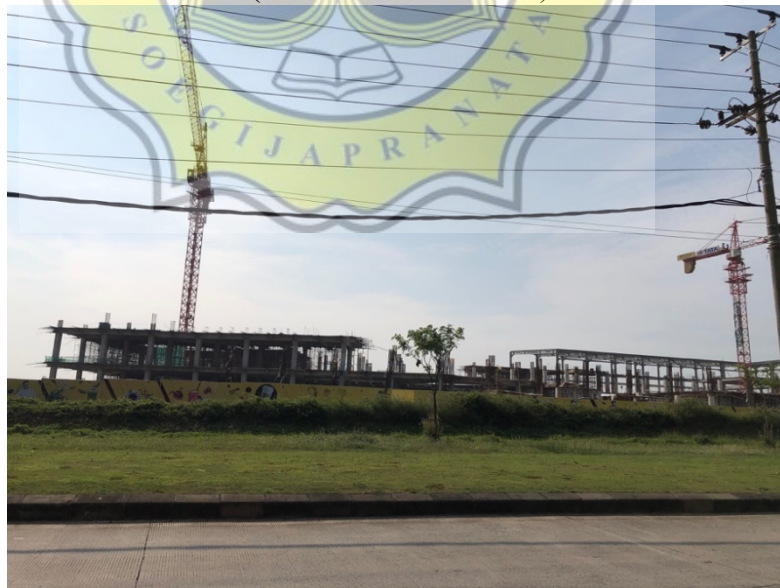
Picture 3.13 A mixed use building is under construction (Mall) Source : personal analysis
