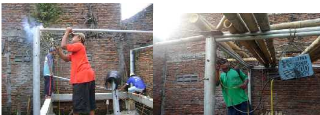
Figure 9: The making and installation of hydraulic pillar made of galvanized pipe (research documentation)
