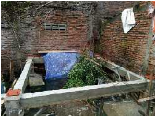
Figure 8: the sloofs used as the building binder for the “Hydraulic House” (research documentation)
