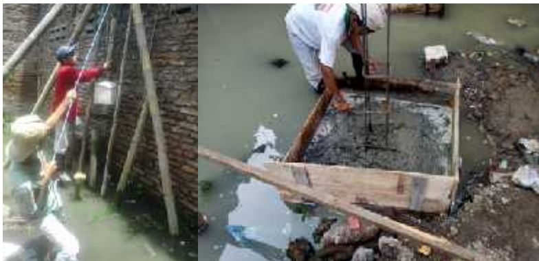
Figure 7: Left: The erection of a bamboo pile as a base for reinforced concrete foundation Right: the making of foot plate reinforced concrete foundation. (research documentation)
