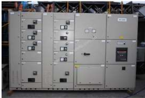
Gambar 5 13 Main Distribution Panel
