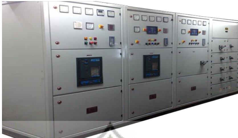
Gambar 7.14. Automatic Main Panel
