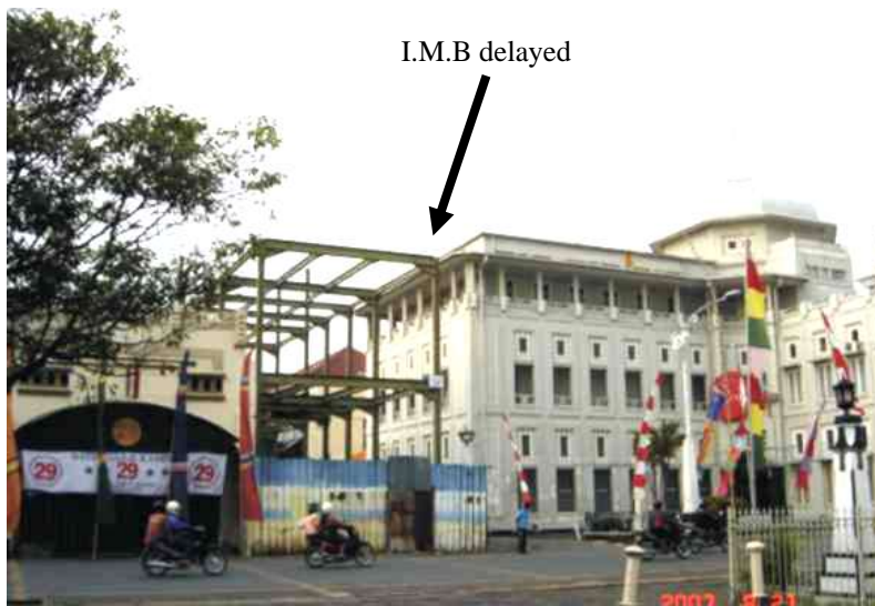
Figure 6 Illegal demolishing of heritage building
