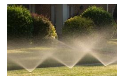
Gambar 3.49 : water sprinkle system Sumber : www.mgf.or.id
