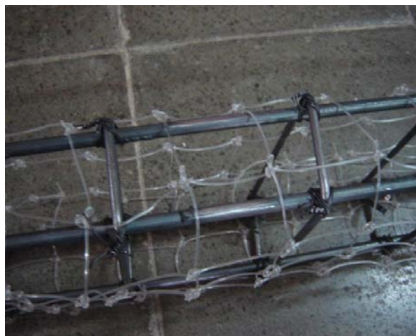
Figure 1. Nylon mesh with mesh spacing of 5 cm which cover the steel bar (Susilorini, 2009b)
