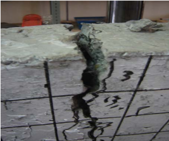
Figure 6. Crack at middle span of beam specimens at ultimate stage (Susilorini, 2009b)
