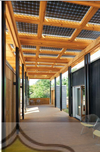
Gambar 74. Atap Photovoltaic Sumber : https://id.pinterest.com/
